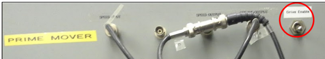
Figure F.5: “Drive Enable” toggle switch on control cabinet
